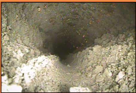
Debris and heavy scale build-up in conduits prior to lining
