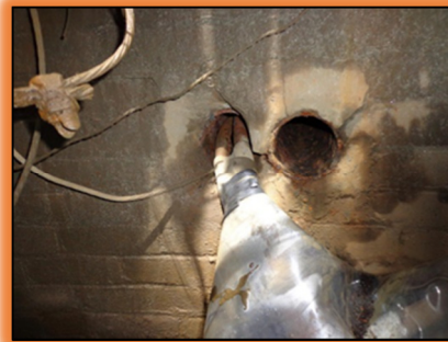
Conduit access inside manhole vault
